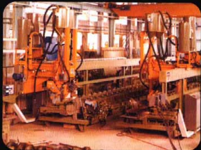
Model 482 Invincible flux recovery systems are mounted high above the work. Each machine serves dual weld heads.
